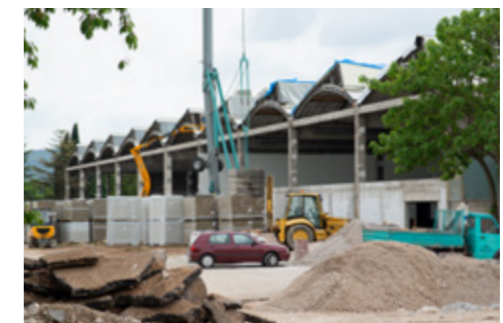
We breath new life in old degraded buildings. We reuse a lot of the construction materials from the demolition work.
